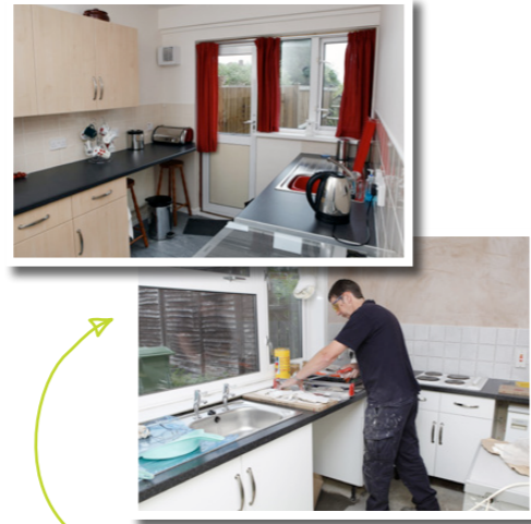
This year we have installed 129 kitchens and 142 bathrooms in our properties. The photos show a new kitchen in Carberry Drive, Portchester and a kitchen being installed in Ransome Close, Titchfield.
