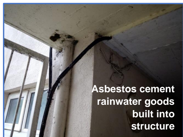
Spalling concrete in stairwell
