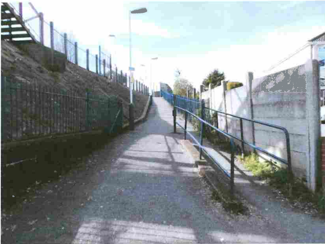
EXIT OR ENTRY NORTH PLATFORM, A VERY STEEP SLOPE
