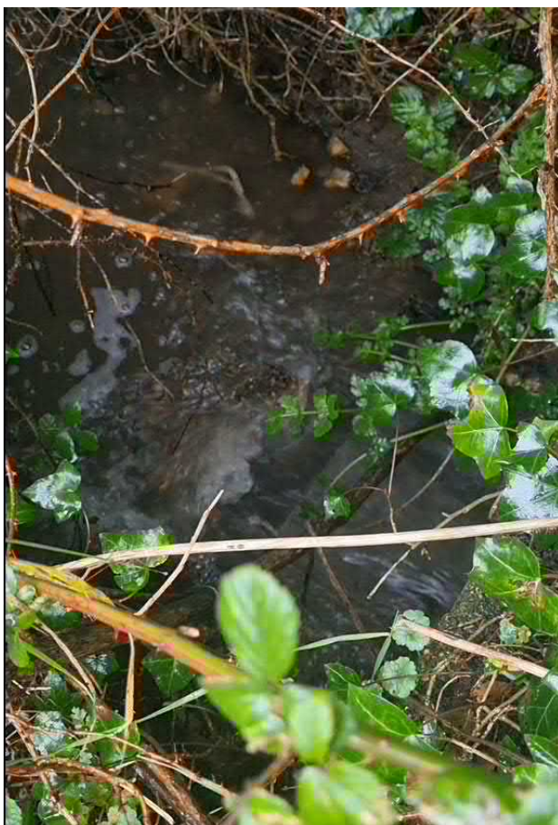
Photograph 3: Culvert outfall to ditch system to the west of the railway bridge.
